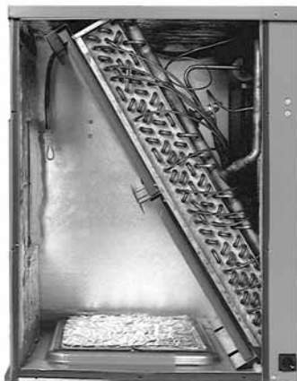
Evaporator Coil/Filter Access
