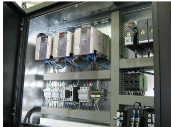
Internally mounted electrical control panel
