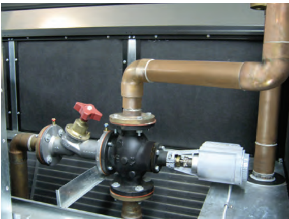
Control valves and piping
