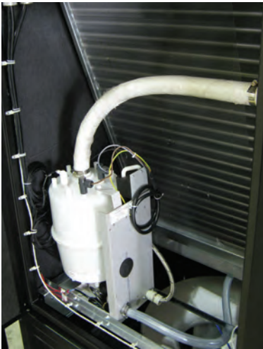
Humidifier and chilled water coil
