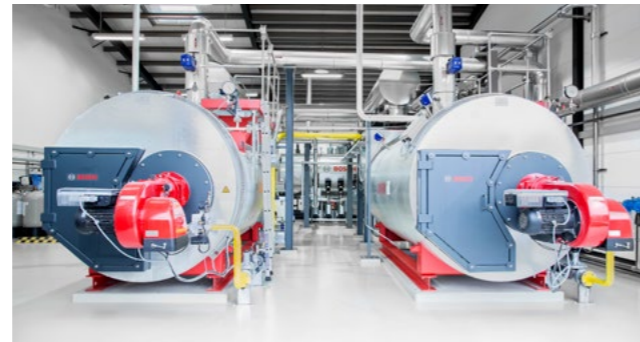
The two efficient Bosch steam boilers supply a total of up to 8 t/h of steam.
