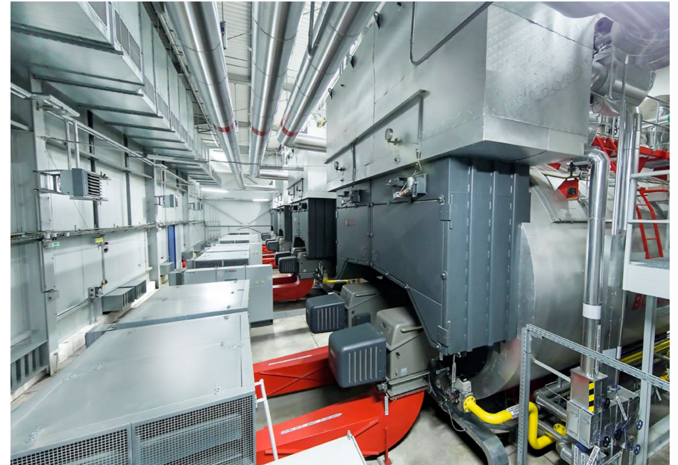
The superheater modules are installed on the front reversing chamber of the boilers.
