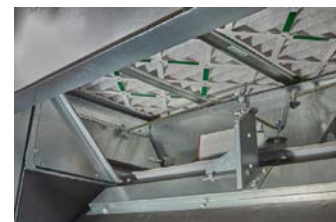
Economizer, Jade Control
