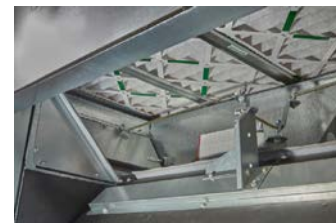
Economizer, No Controls
