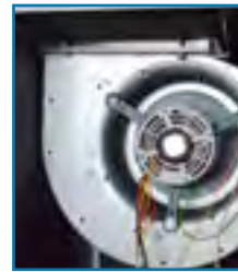
Interior of Supply Fan Section
