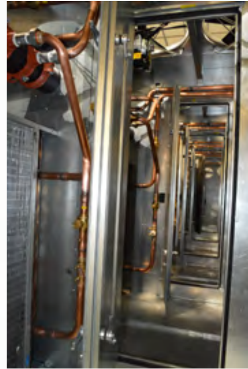
▲ Walk-in Service Access
