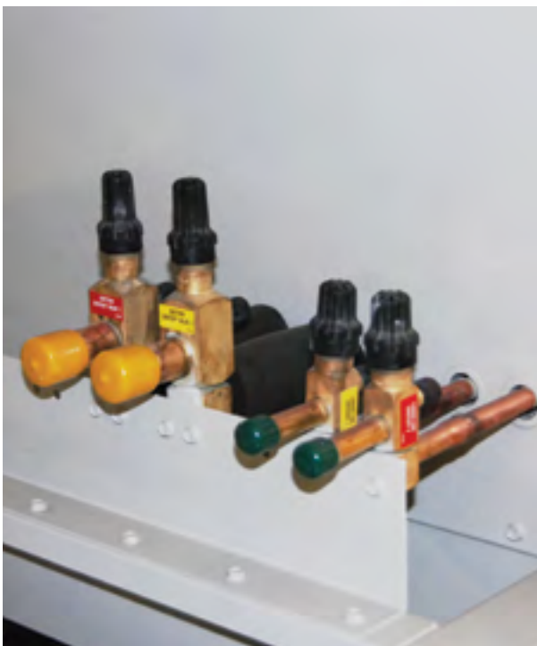
Split system copper stub outs with shut-off valves are easily accessible outside of the cabinet.
